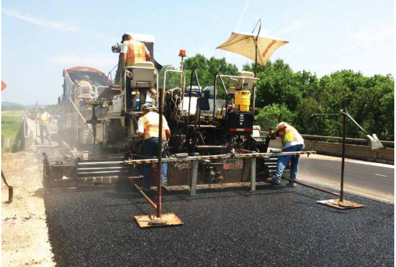
NMC supplied 750 tons of dry scrubber ash for this stone matrix asphalt paving project on I-94 in central Wisconsin.
